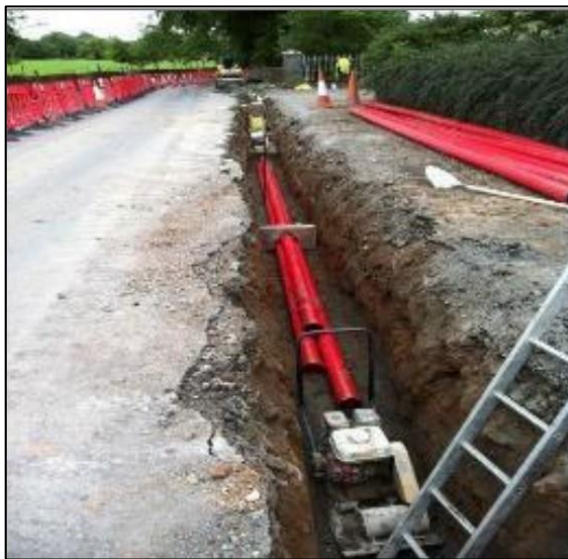
Figure 2-3: Typical 110kV Installation (Source: TLI Group)
